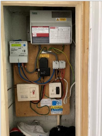
Photo 38 Unmodernised electrical equipment
