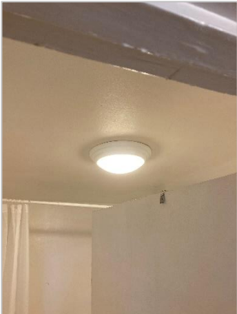
Photo 40 Surface mounted fitting in bathroom
