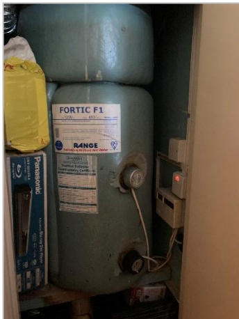
Photo 21 Typical cold water tank and hot water cylinder
