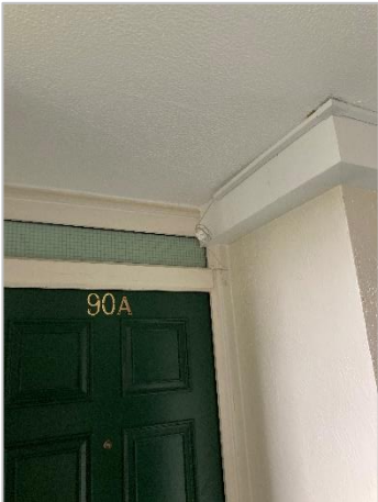
Photo 18 Some loose cabling
