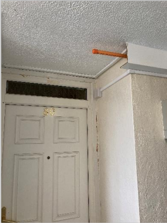
Photo 13 Flat 80 not connected to sprinkler system?
