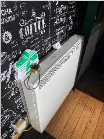
Photo 39 Newer storage radiator
