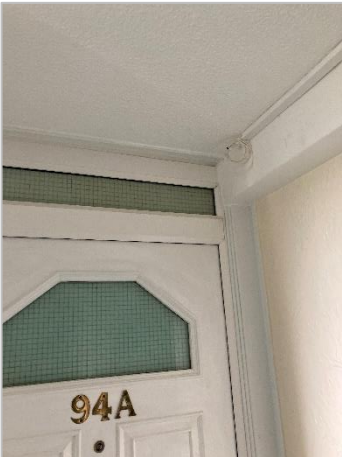
Photo 17 Some loose cabling
