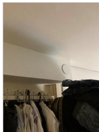
Photo 24 Residential sprinkler system concealed head
