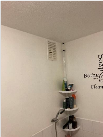
Photo 35 Poor bathroom extract ventilation
