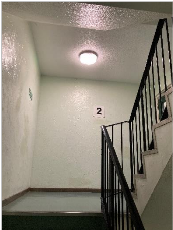
Photo 10 Newer staircase emergency light
