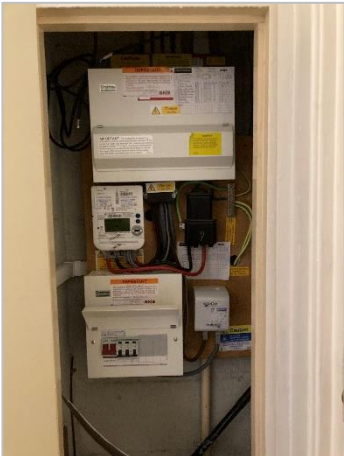
Photo 32 'Modernised' electrical equipment
