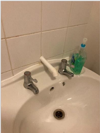
Photo 30 Overflow from hot water cylinder/tank
