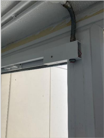
Photo 8 AOV actuator cover missing
