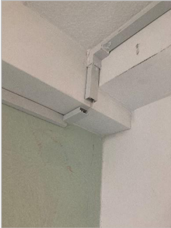
Photo 7 Damaged smoke cable trunking
