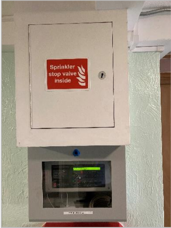
Photo 4 Sprinkler control panel
