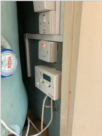
Photo 28 Typical hot water cylinder heater controls
