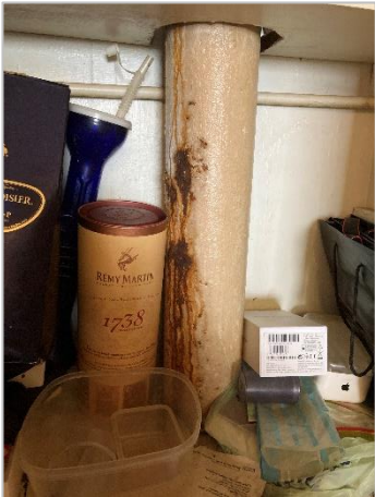
Photo 34 Apartment 90A leaking soil stack
