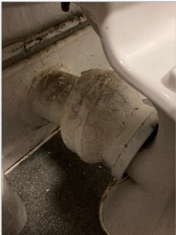
Photo 36 Original cast iron drainage leaking
