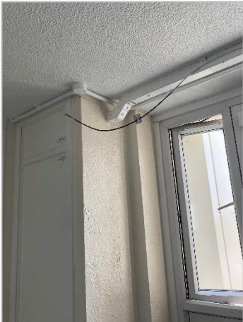
Photo 16 Some loose cabling
