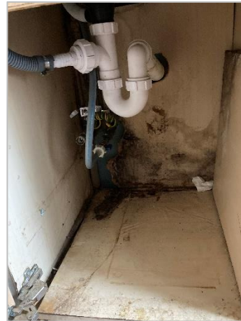
Photo 20 Evidence of leak under sink (28A)
