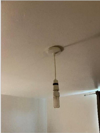
Photo 25 Typical pendant light fitting
