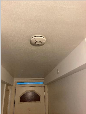
Photo 26 Smoke detector in entrance lobby
