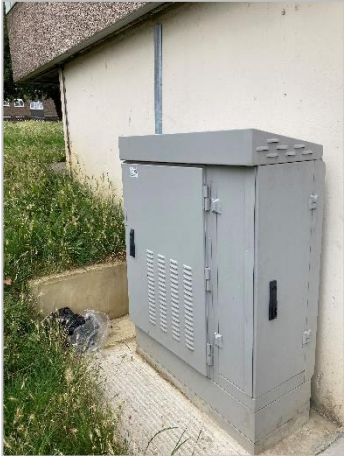
Photo 14 New incoming telecommunications
