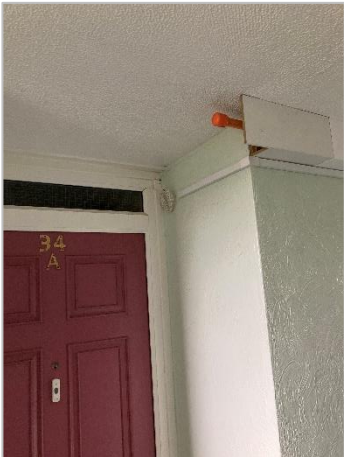
Photo 12 Flat 34A not connected to sprinkler system?
