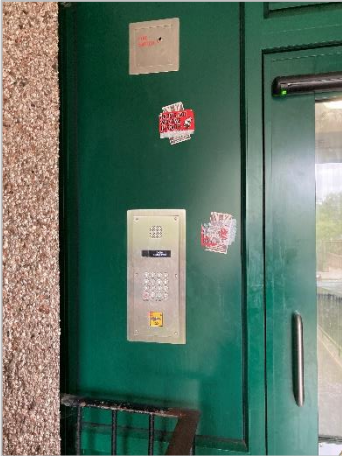
Photo 1 Door entry and access control panel
