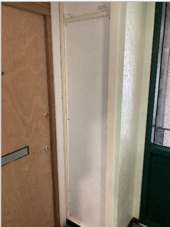
Photo 5 Apartment electrical cupboards have been sealed shut
