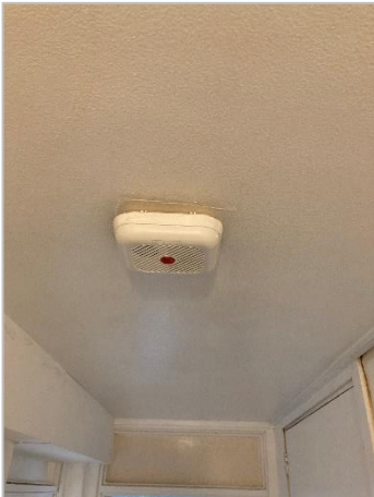
Photo 31 Older smoke detector
