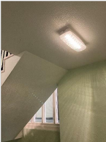
Photo 11 Older style staircase light
