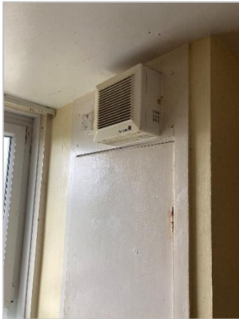
Photo 19 Typical kitchen extract fan
