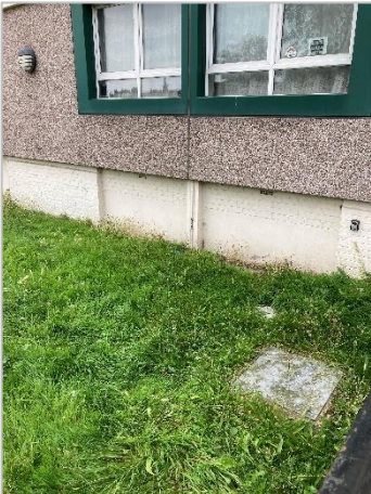
Photo 15 External lighting and earthing tape
