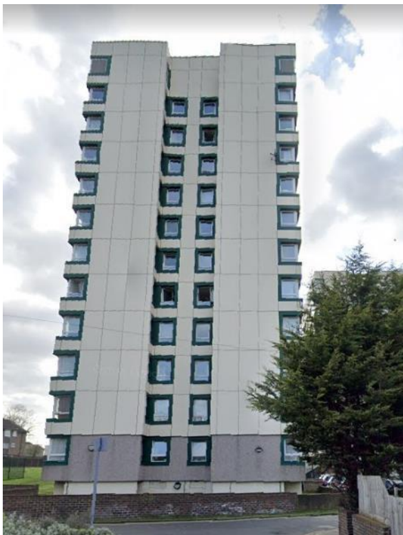
Fig 5 Western elevation 58-108A showing render finish to ground floor to over-cladding and aluminium panels used for remainder of block
