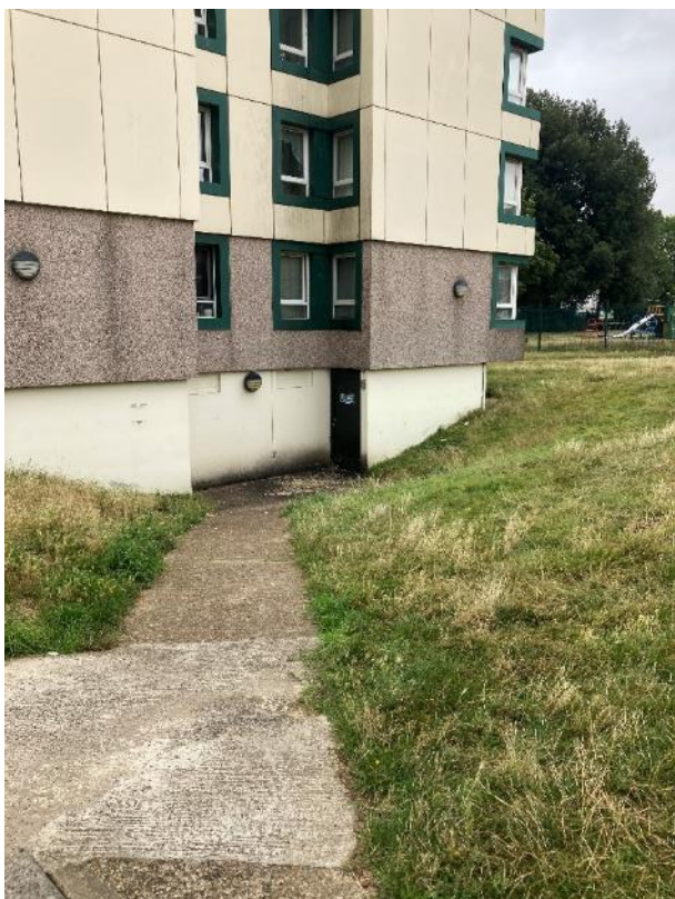
Fig 7 Eastern elevation 58-108A Showing render finish to ground floor to concrete and brick substructure
