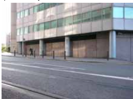
The ground floor of this office has no windows or doors. It is an attractive opportunity for vandals.
