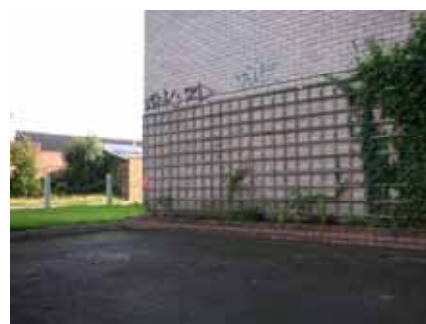
Textured surfaces, intended to disrupt the overt impression of the paint is one way of tackling graffiti. In this example trellis was added but only worked as a deterrent to graffiti where there was planting too.
