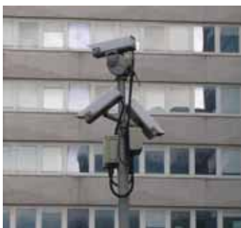
Cameras must take account of the context, as they can add to visual clutter in the street scene. Whilst they can give reassurance, the obvious presence of cameras can add to the perception that crime is present.
