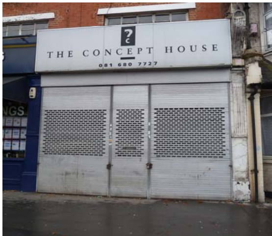
Unacceptable a mix of solid and open grille design external shutter
