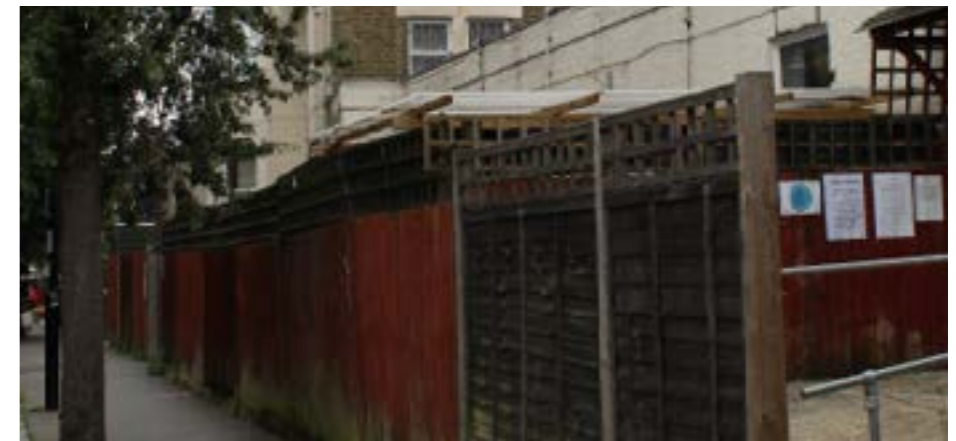
134. Loss of historic boundary treatments and use of modern materials for boundary walls
