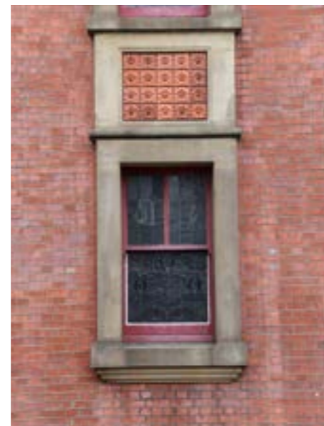
92. Red brick with stone and tile details, with sash window and stained glass (Stanley Halls)
