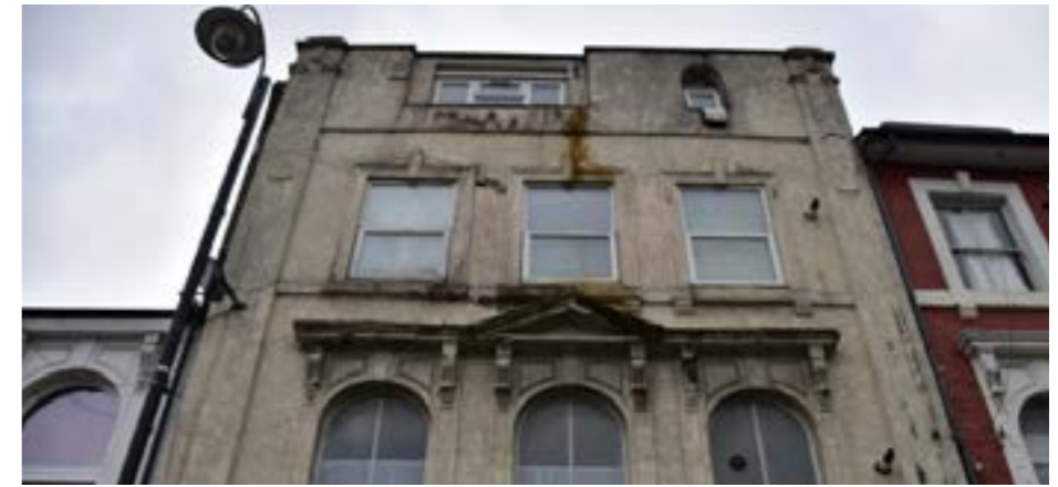
133. Example of the threat caused by lack of routine building maintenance
