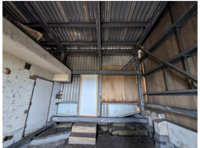
Figure 18: Internal wall and ceilings of the annexe
