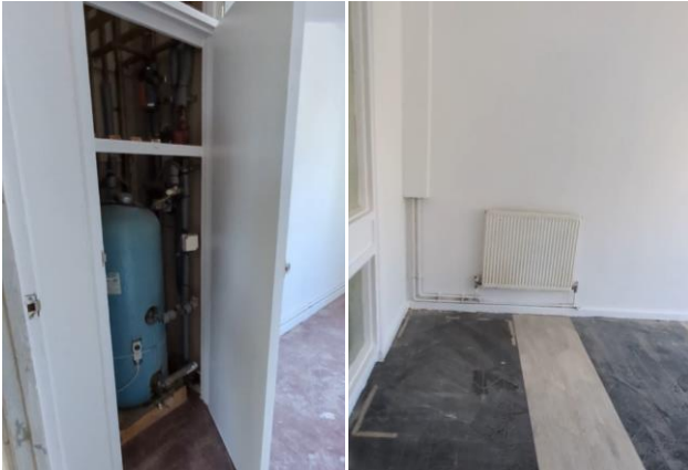
Figure 27 & 28: Gas boiler and radiators within the units
