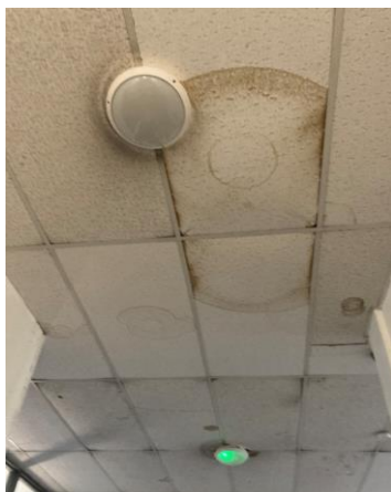
Poor condition of suspended ceilings in hallway
