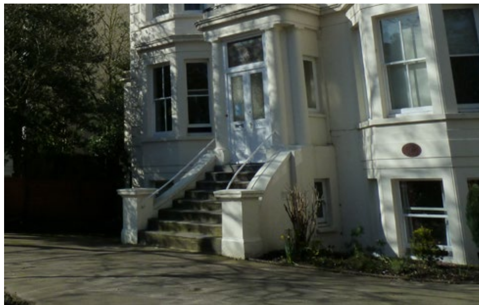
Originally an open porch with free standing columns and infill that has been enclosed, harming the appearance of the property
