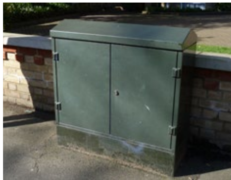
Well sited telecommunication cabinet to the rear of the footway
