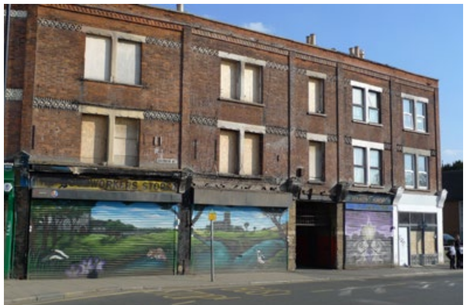
105-109a Church Street (locally listed), fire damaged and mostly vacant
