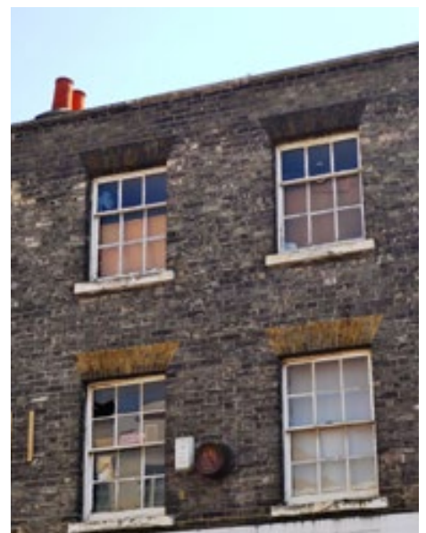
Poorly maintained timber sash windows and cills
