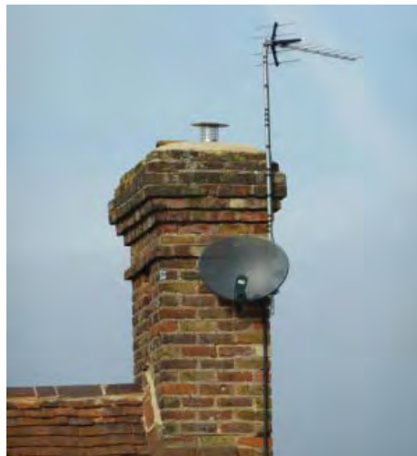
Poor location of equipment
