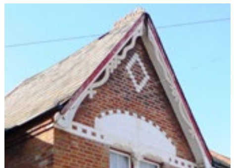
(Above) Victorian Terraces Character Area: Some examples of material and architectural details present
