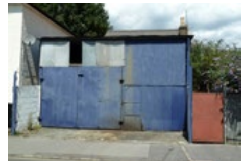
2A Howley Road, which detracts from the character of the conservation area
