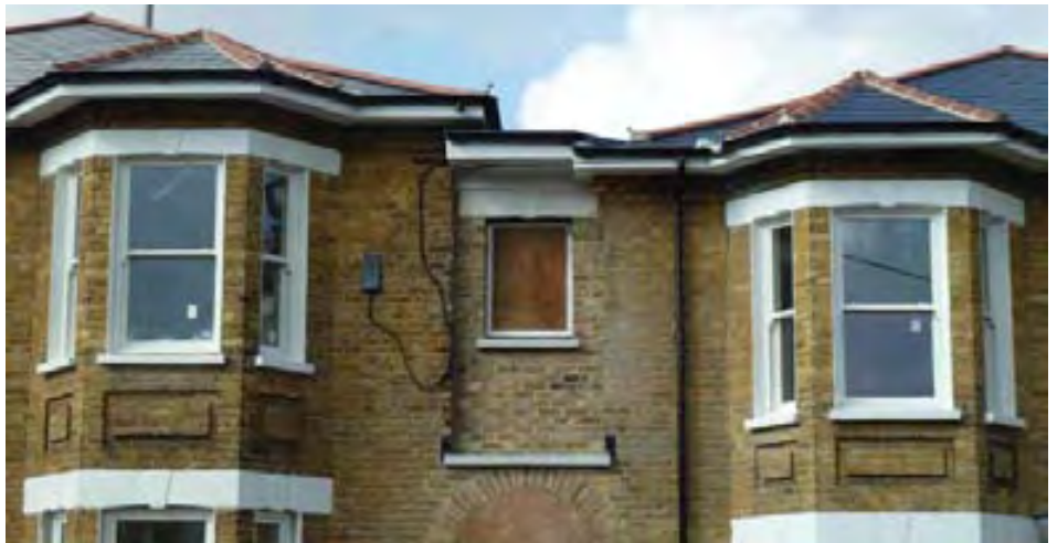
Example of poorly executed conversion combined with conjunction of buildings
