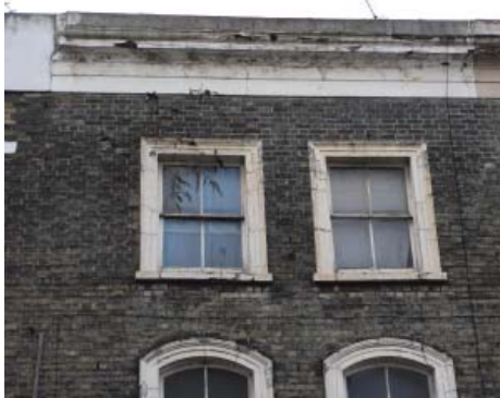
Victorian buildings in a poor state of repair
