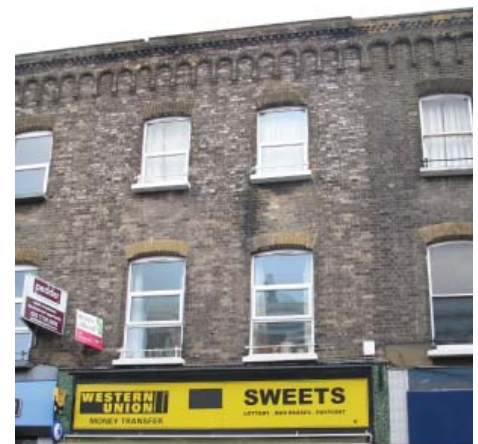
Unauthorised replacement uPVC windows that have had a negative impact on the character of the host building, which would originally have had timber sash windows
