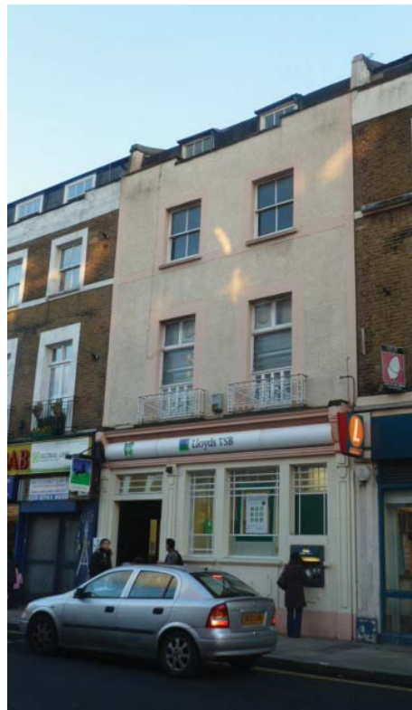
Inappropriate render applied to a building on Westow Hill that has harmed the unity of the terrace
