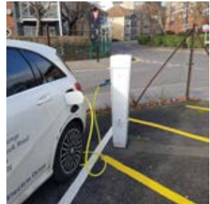
Vehicle charging points in Wandle Road car park
