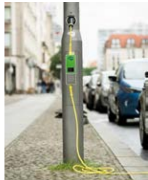
Vehicle charging point fitted in lamp column
