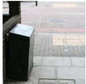
Utility cabinet located at the rear of the street, painted black
