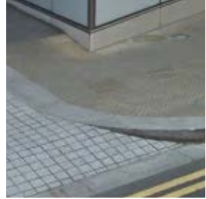
Precise detailing at vehicle crossovers can allow to minimise extent of the crossfall change
