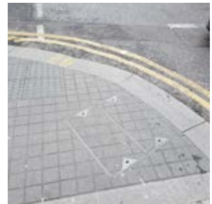
Areas of footways along Lansdowne Road where vehicular overrun was anticipated were treated accordingly with granite setts
