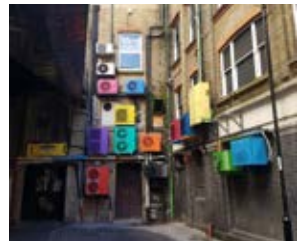
Art to deal with unsightly conditioning units along Surrey Street
