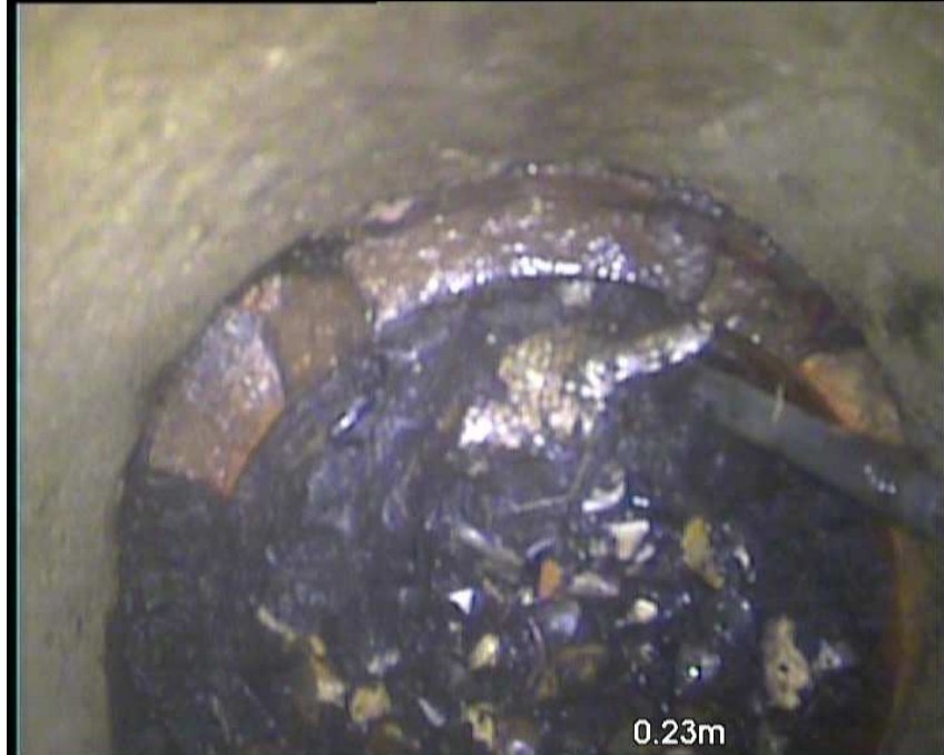
Photo: 0000005.jpg, 00:00:00 0.53m, Collapsed drain/sewer
