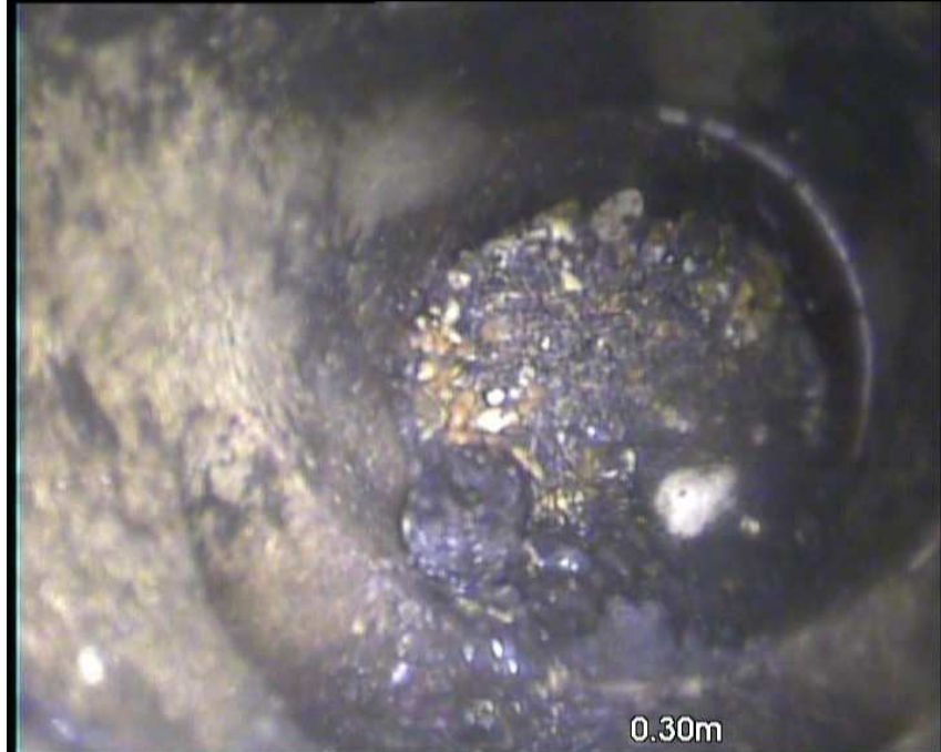
Photo: 0000006.jpg, 00:00:00 0.5m, Collapsed drain/sewer
