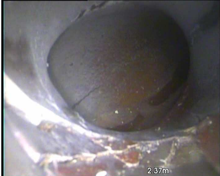
Photo: 0000003.jpg, 00:00:00 2.37m, Fracture, multiple, from 7 to 9 o'clock
